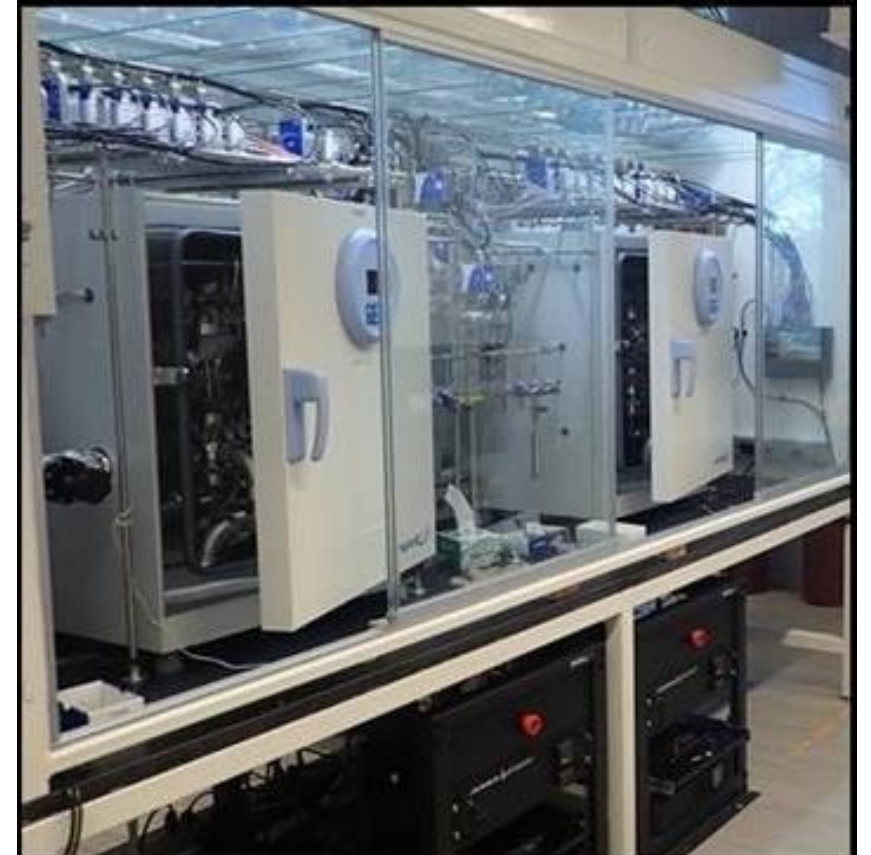
The two new ALD reactors in the vented enclosure. The substrate heater controls are visible underneath the enclosure
